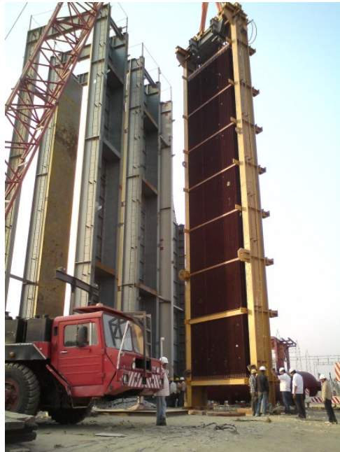
The installation of a HRSG for a gas based combined cycle power plant in northern India
