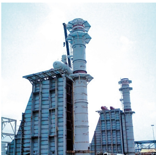
Greens' premium HRSGs for a gas based combined cycle power plant in northern India
